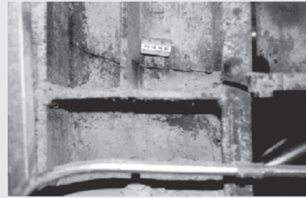
(b) Fracturing of W14 column at welded beam-to-column connection in Northridge earthquake
